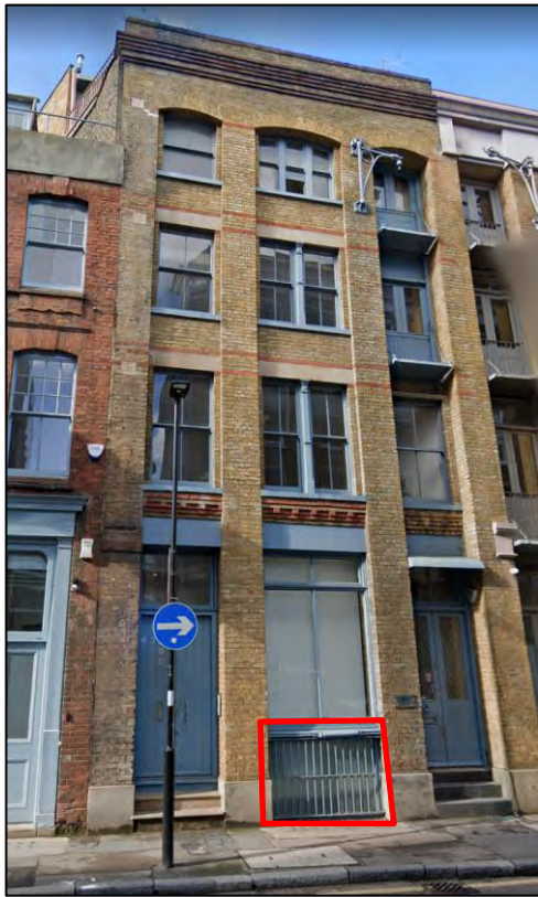
Figure 35: 43 Tabernacle Street, the impacted window is outlined in red.
